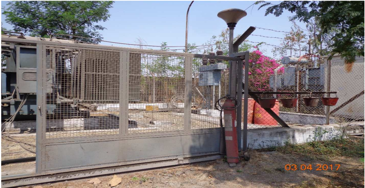
Switch yard station
