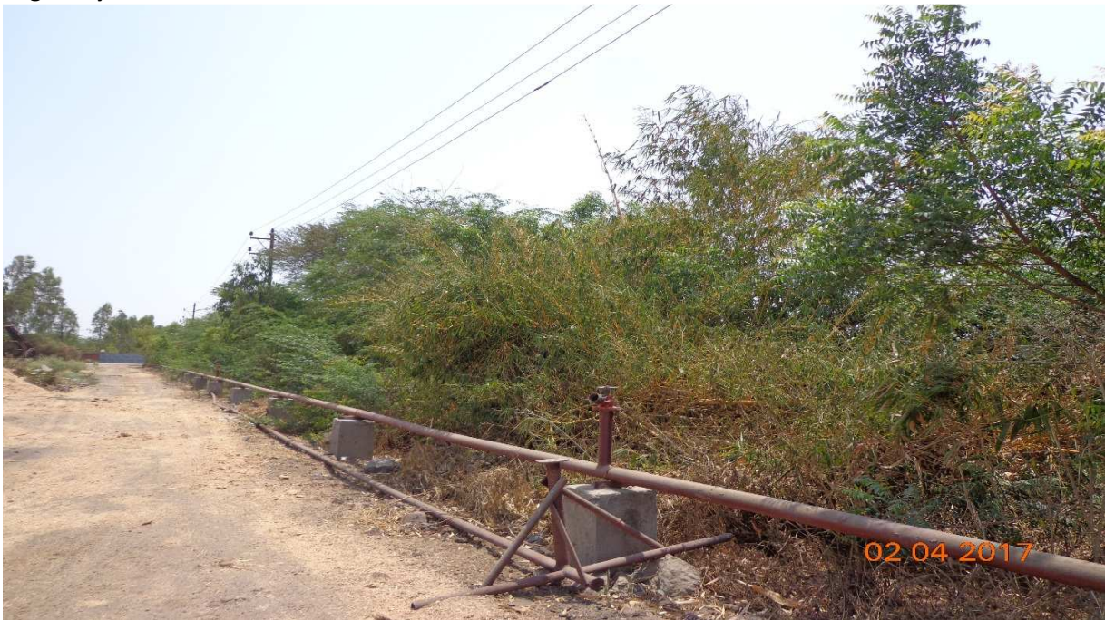
Bagasse yard fire line
