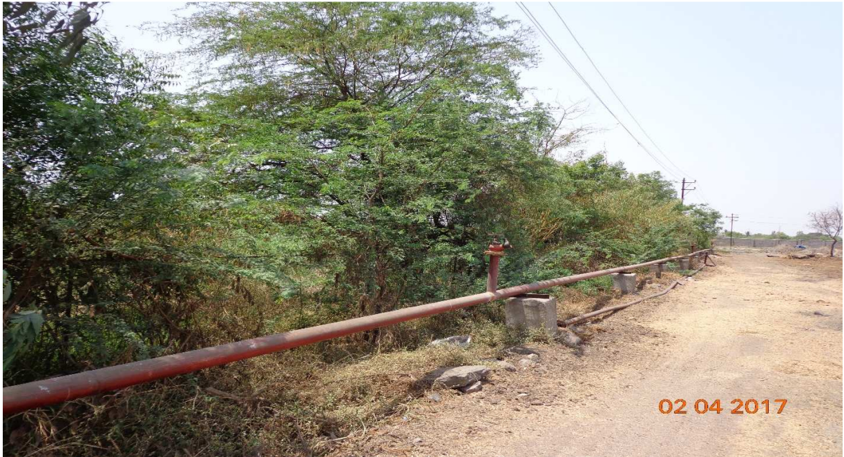
Bagasse yard fire line
