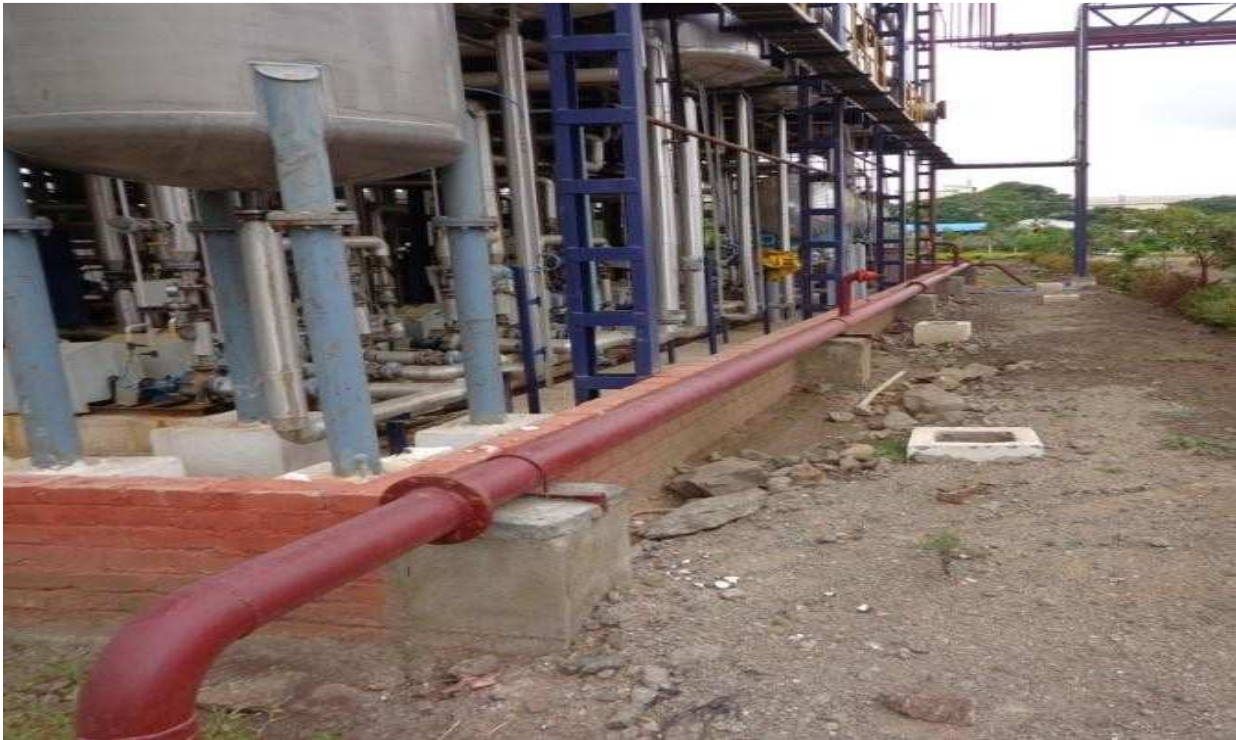
Fire hydrant system
