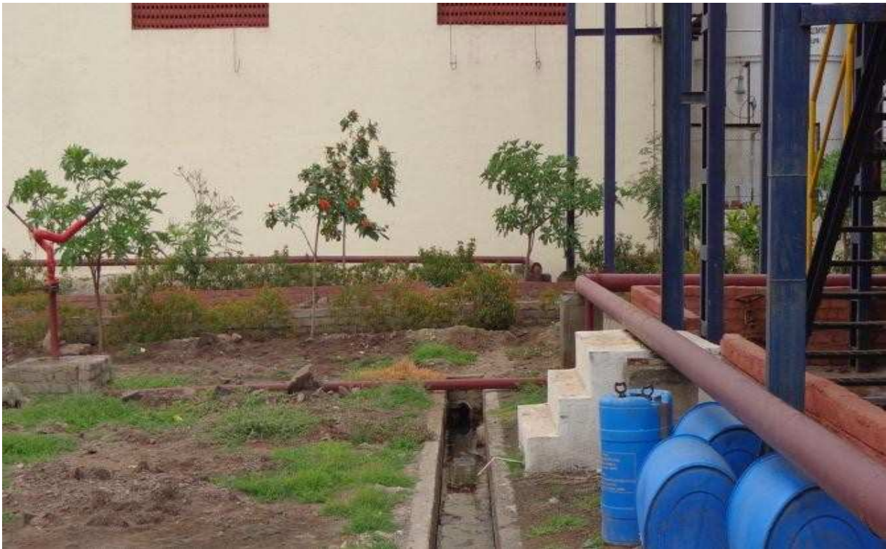
Fire hydrant system
