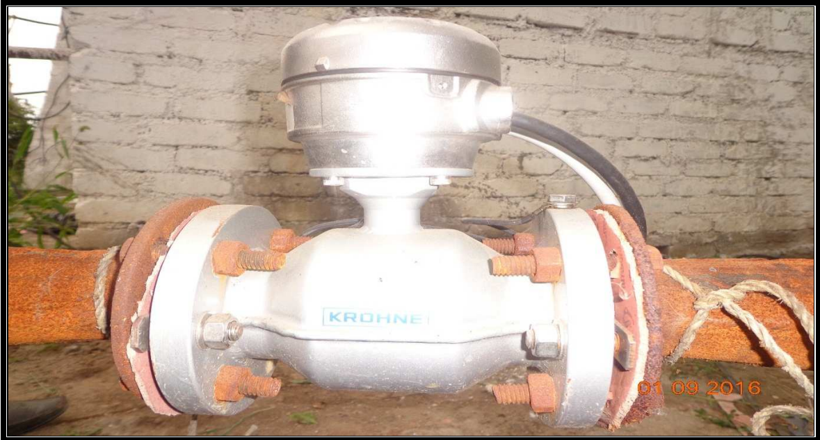
Water Flow Meter
