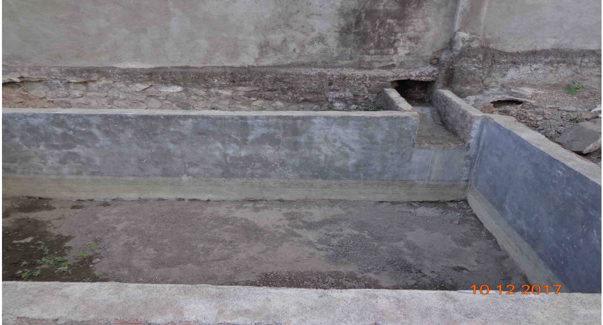
Rain water Near sugar godown collection tank
