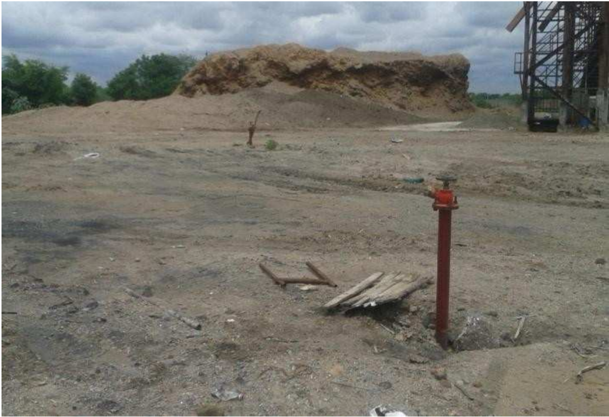
Bagasse yard fire fighting system
