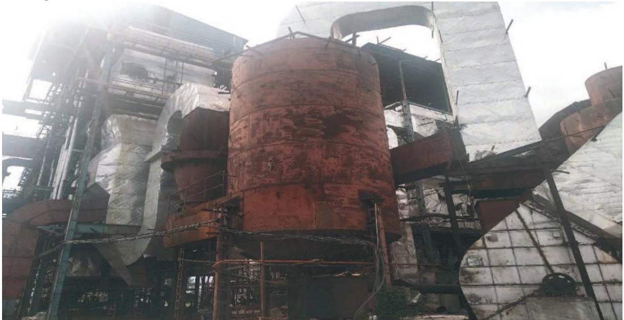
Existing Venturi wet scrubber
