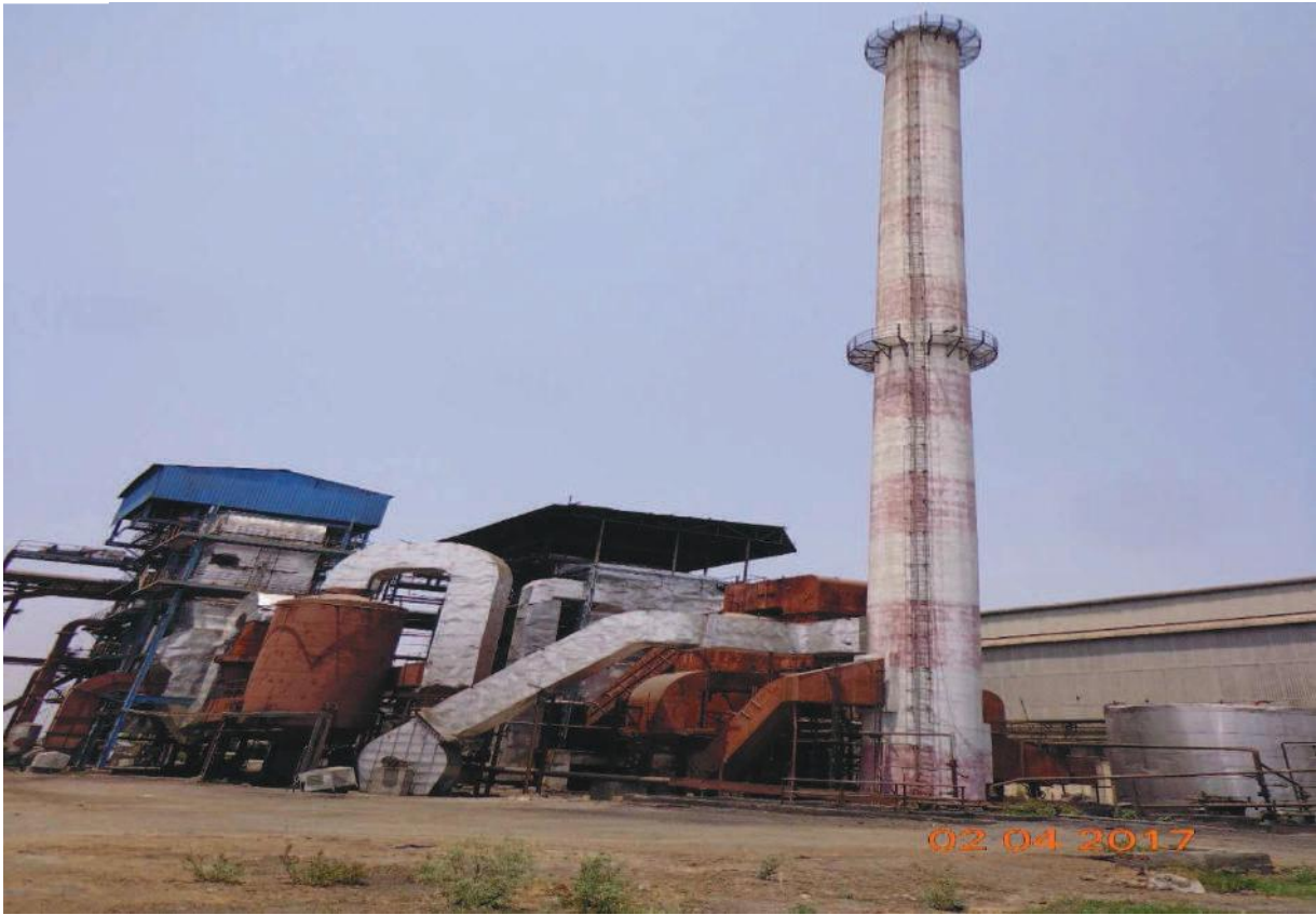
Existing Boiler 70 TPH & 32 TPH & Stack
