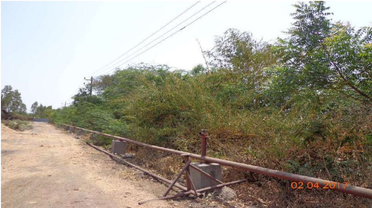
Bagasse yard fire line
