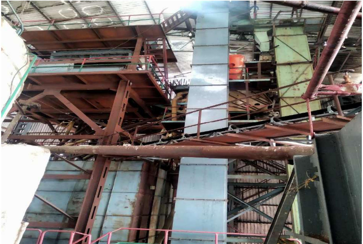
Sugar grader & Sugar elevator added
