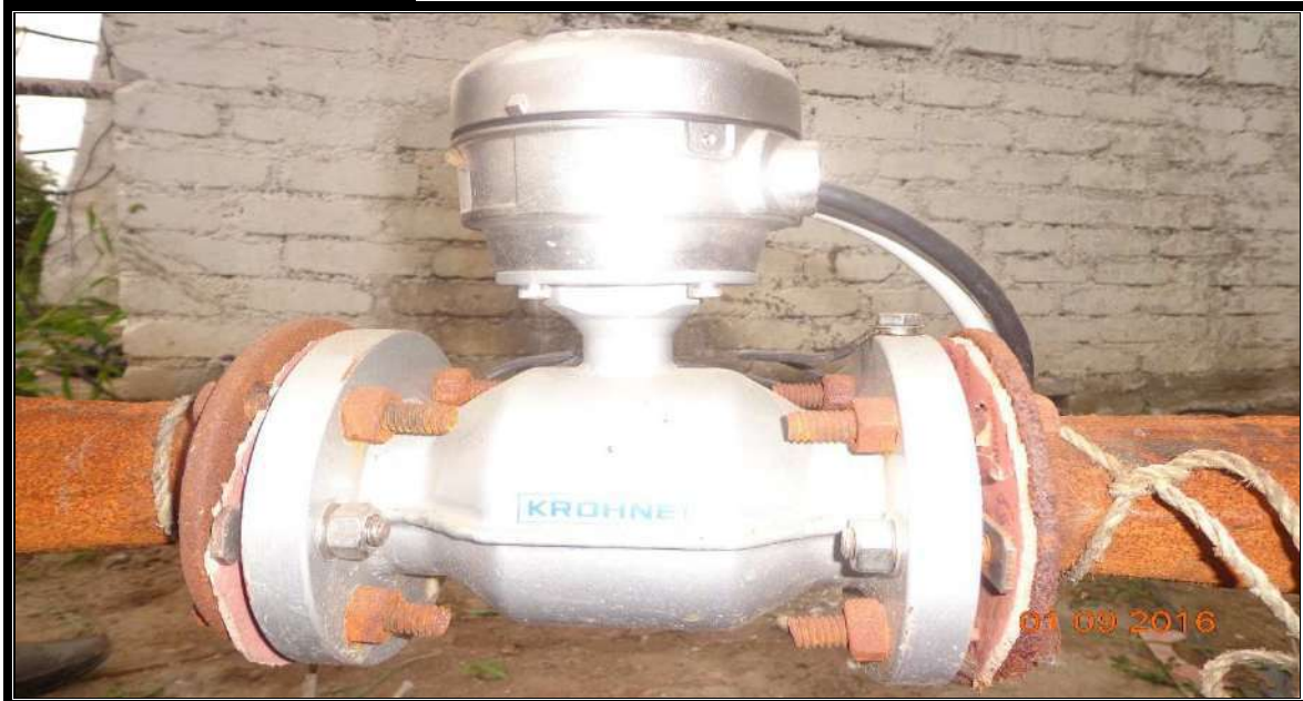
Water Flow Meter
