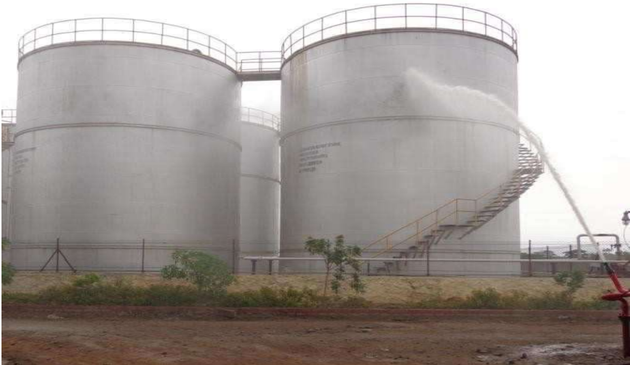
Fire hydrant system
