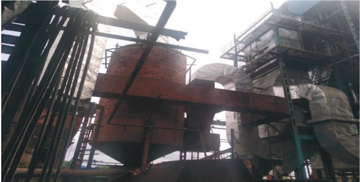
Existing Venturi wet scrubber
