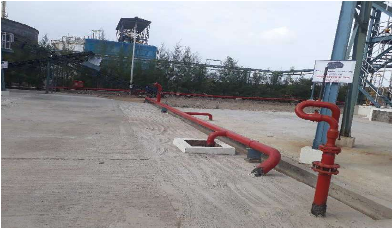
Fire fighting system
