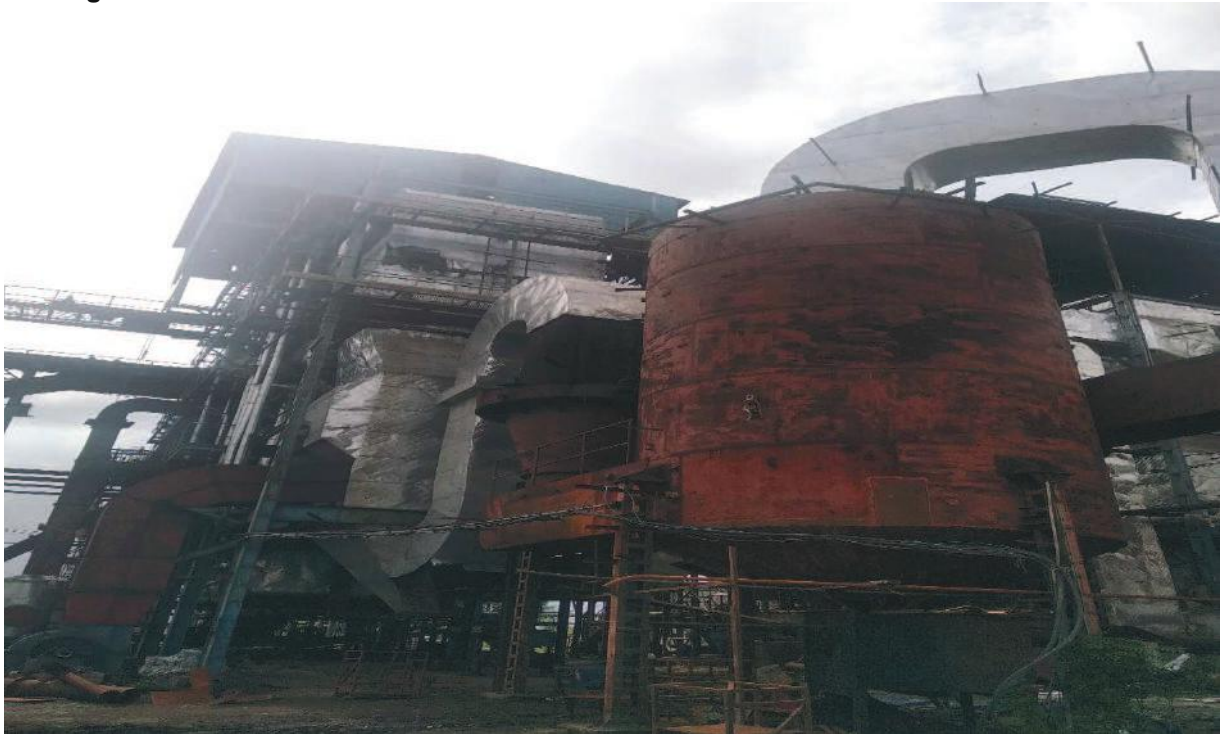
Existing Venturi wet scrubber
