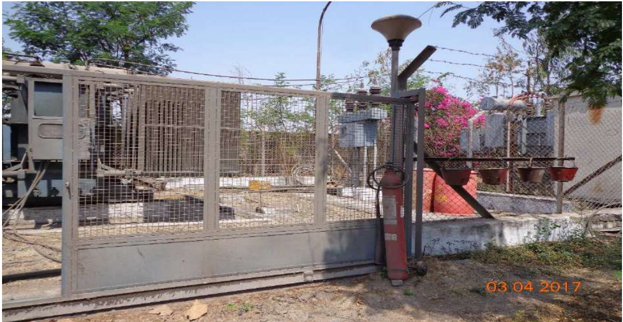
Switch yard station
