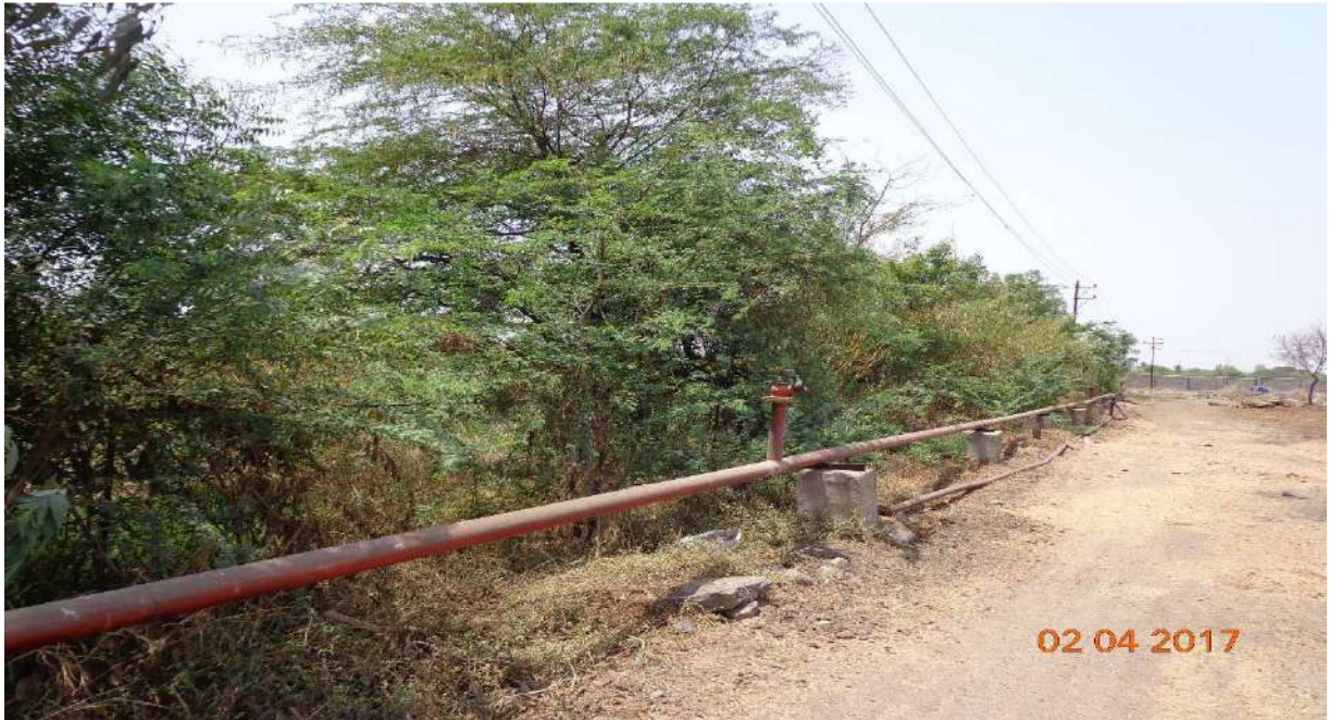
Bagasse yard fire line
