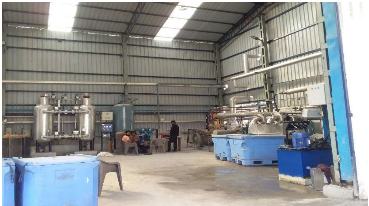
CO2 Processing & Bottling Plant at Shreenath Mhaskoba Sakhar karkhana Ltd.,
