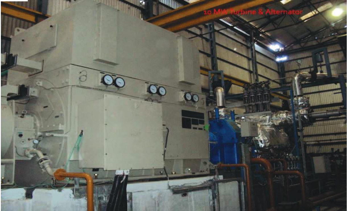
Existing 10 MW Turbine & Alternator
