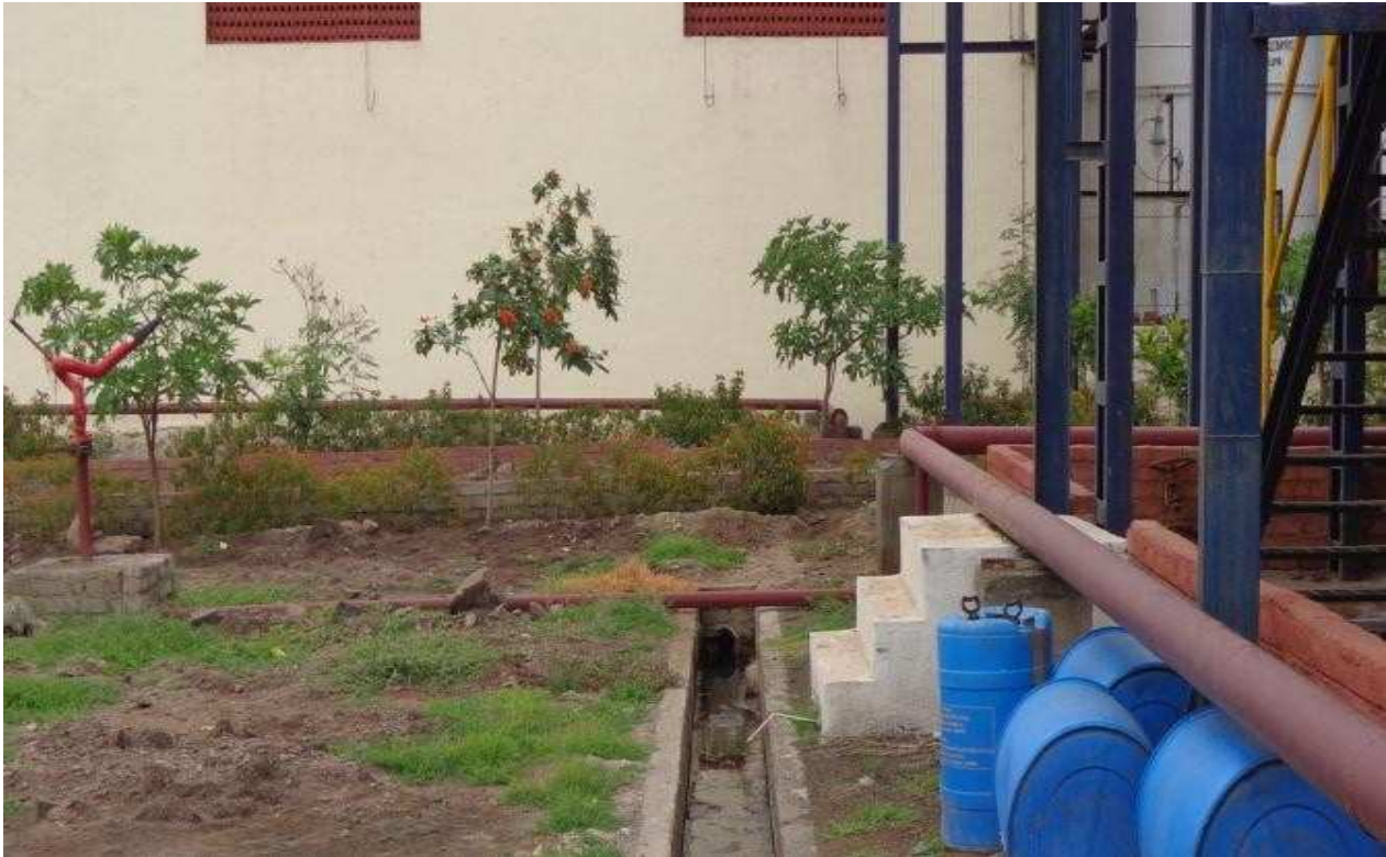
Fire hydrant system
