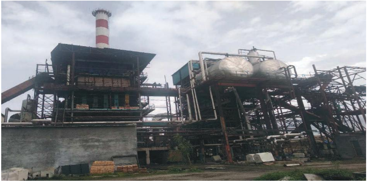
Existing Boiler 70 TPH & 32 TPH
