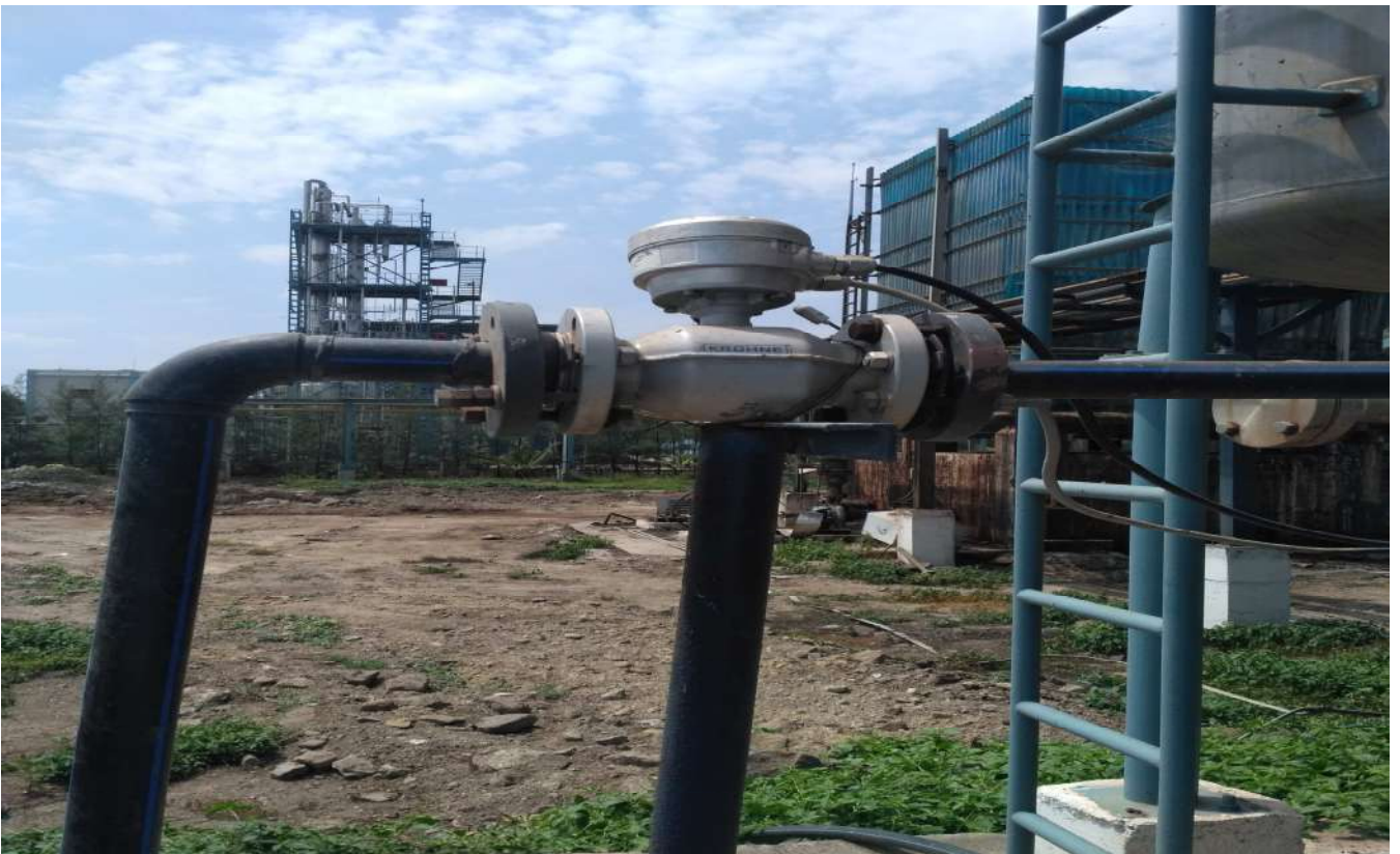
Image 2 : Magnetic Flow Meter
