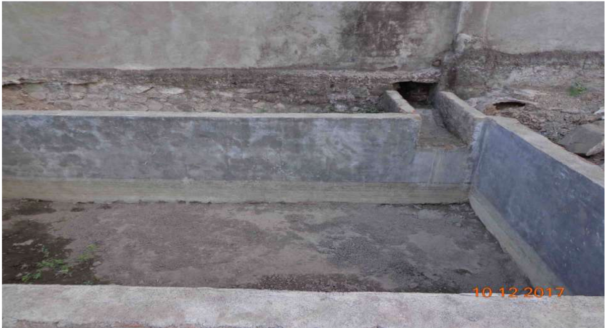
Rain water Near sugar godown collection tank
